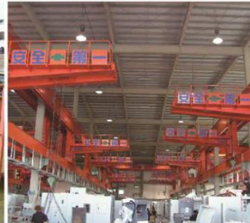
2006 Paterson Machinery 3 tons jib crane with 9M height
